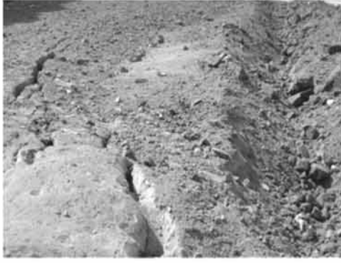
3 Test no. 1, crack propagated behind pre-splitting row
